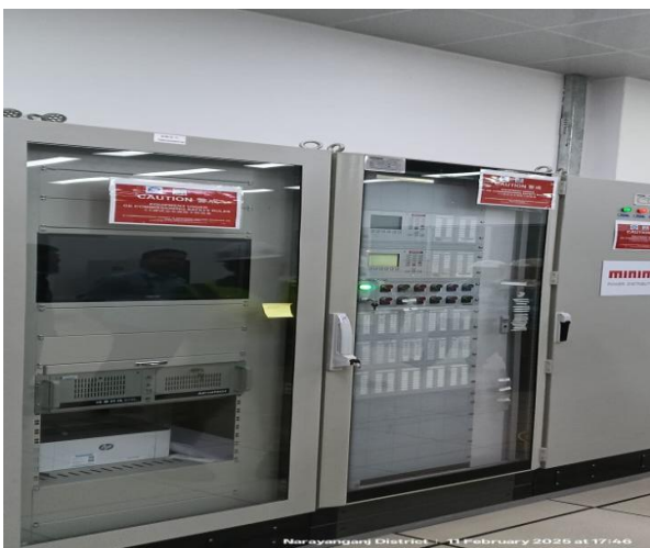
Photo 5: Fire control panel in CCB room
