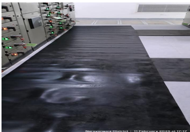
Photo 2: Insulation mat provided in front of electrical panel
