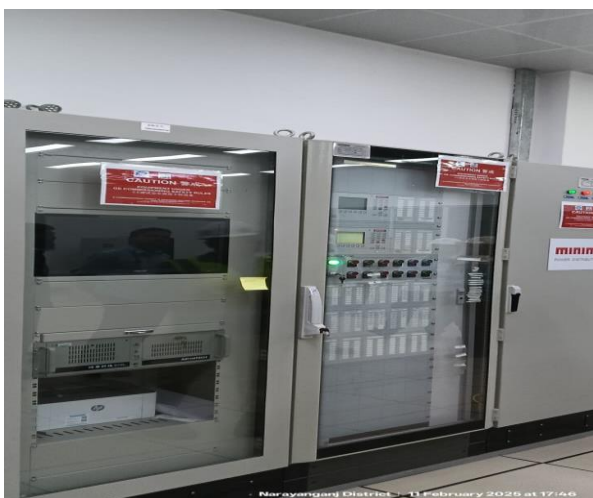
Photo 5: Fire control panel in CCB room
