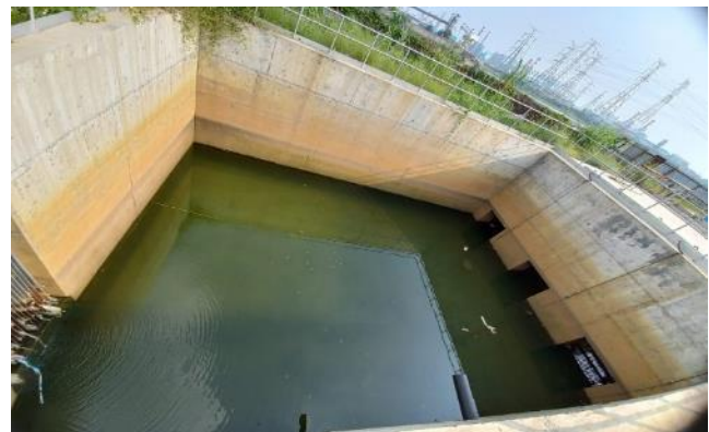
Photo 12: Treated Effluent Storage Basin
