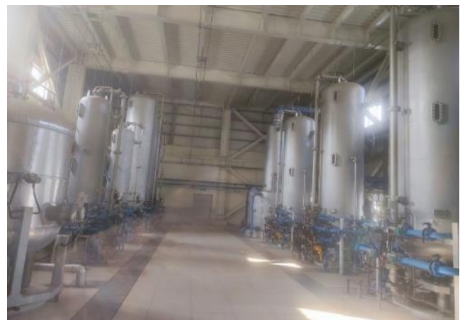
Photo 10: DM Water Plant
