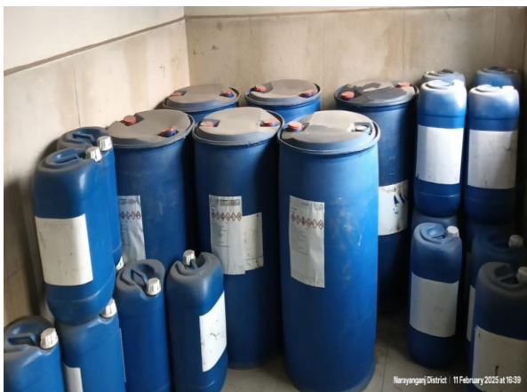
Photo 3: Aqueous Ammonia stored in steam turbine building
