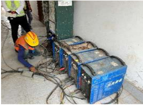
Fig 1: Insulated mats not provided for the arc welding machines
