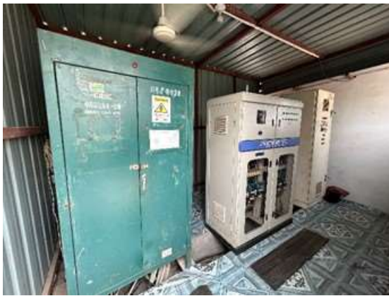
Fig 15: Smoke detection system not installed at the electrical panel room at worker camp
