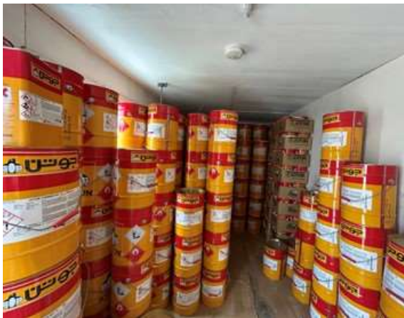
Fig 17: Chemical compatibility matrix and flame proof electrical fittings lacking at paint and thinner store at worker camp
