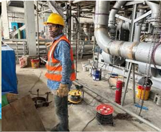
Fig 12: Fire watch and appropriate PPEs viz welding helmet missing for worker involved in hot work
