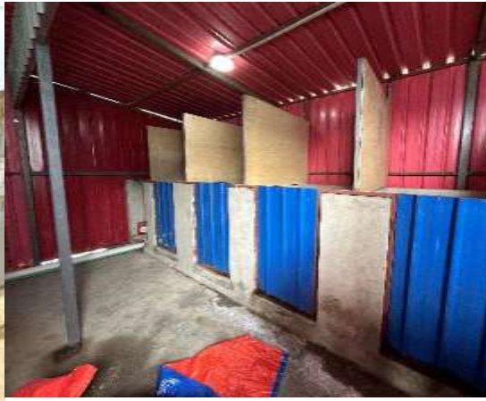
Fig 10: Privacy lacking at the sanitation facility provided for the driver accommodation
