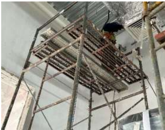
Fig 3: Make shift toe boards do not conform to BNBC requirements
