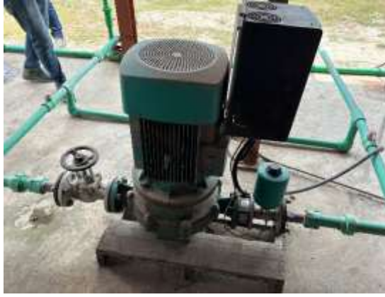
Fig 16: Electrical motor of the water treatment plant is not provided with dual earthing
