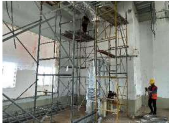
Fig 2: Scaffold lacking inspection tags
