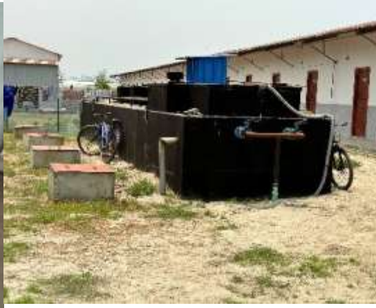
Fig 8: Operational STP installed at worker camp
