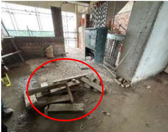
Fig 7: Missing fire extinguisher near panel; flammable wooden plank stored near panel
