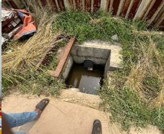
Fig 18: Storm water drains not subjected to cleaning & maintenance
