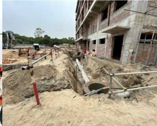
Fig 6: Missing barricading at excavated trench near dormitory building
