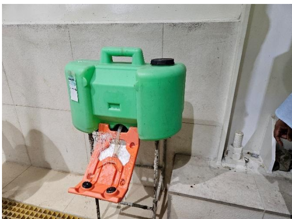
Photo 1: Eyewash in Chemical Dosing Room in DM Plant
