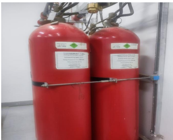
Photo 7: Gas suppression system in DM water building control room
