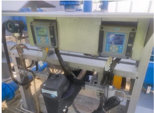
Photo 14: Online effluent quality monitoring
