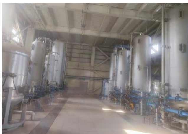
Photo 10: DM Water Plant
