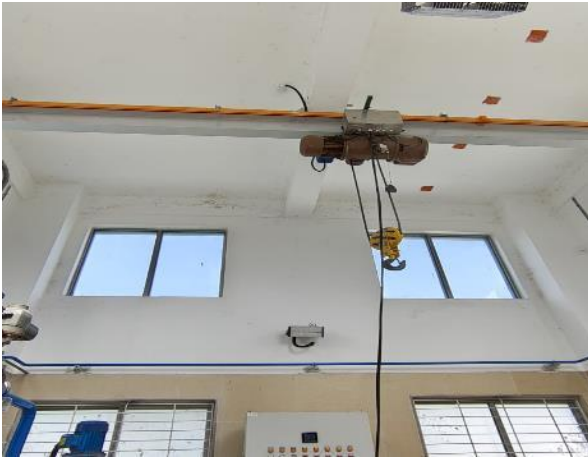
Photo 13: Multi Detector installed in Hypo chloride doing building
