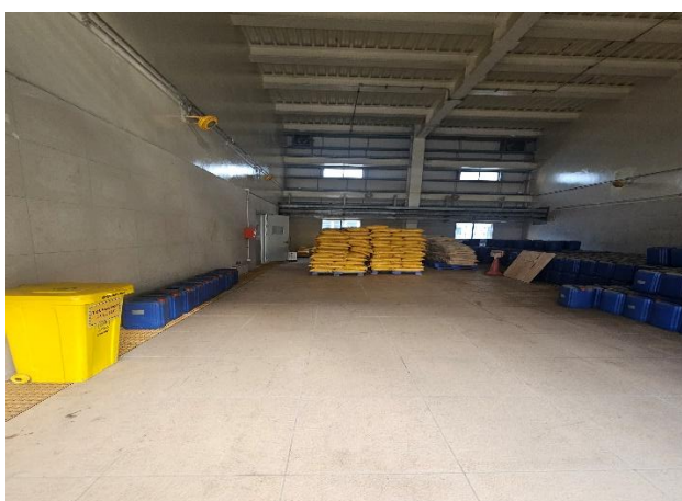
Photo 4: Chemical storage room for DM water plant
