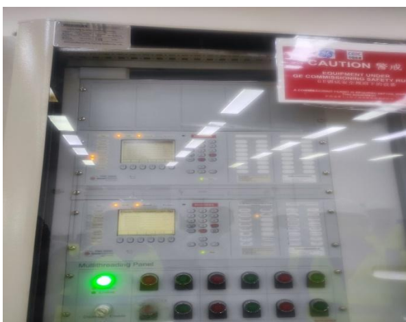
Photo 5: Fire control panel in CCB room
