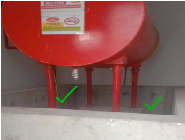
Photo 7: Double Earthing provided at Fire Diesel Tank storage.
