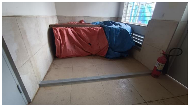
Photo 6: Secondary Containment at Hydrazine Storage
