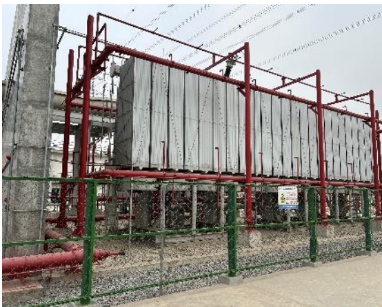
Photo 11: Automated fire suppression system installed at the transformer area
