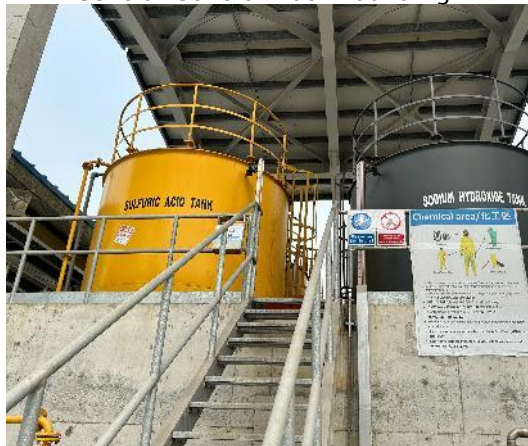
Photo 4: Acid and alkali storage tanks onsite
