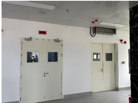
Photo 2: Provision of emergency exit signages and fire rated doors at the Central Control Room building
