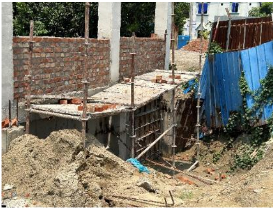
Photo 15: Unstable platform and damaged scaffolding for work at height
