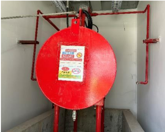
Photo 7: Diesel storage tank at fire pumphouse without earthing and overflow protection
