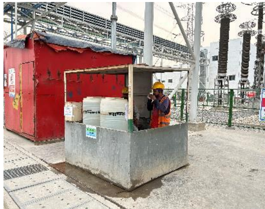
Photo 16: Rest rooms with drinking water provision onsite
