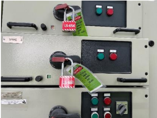
Photo 13: LOTO system implemented in electrical panel
