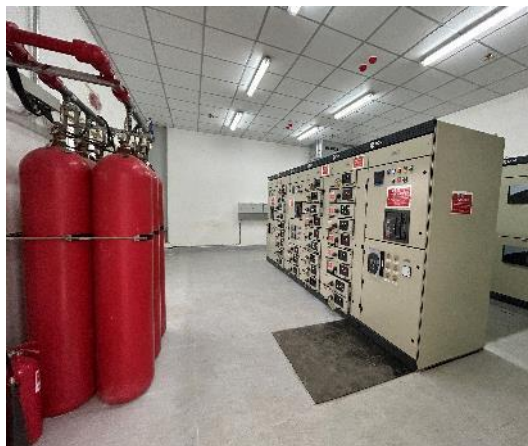
Photo 12: Automated fire suppression system at the electrical panel room
