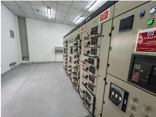
Photo 19: Missing insulated mats at the electrical panel room
