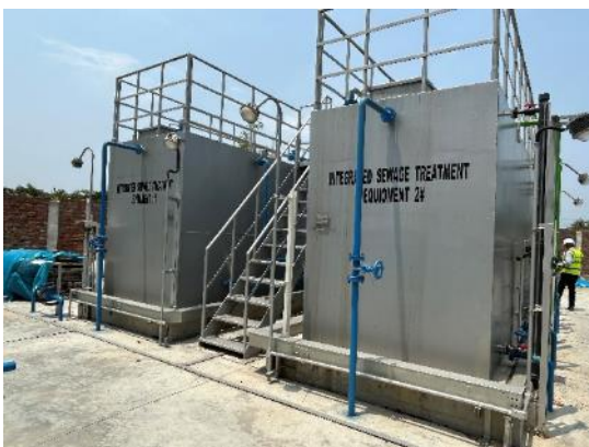
Photo 17: STP in operation at site
