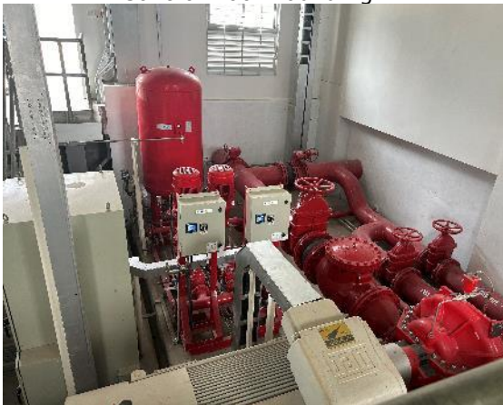
Photo 3: Fire pump room onsite
